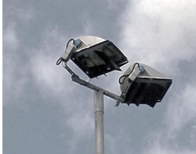
Artificial (Flood) Light Mast with Two Luminaires and Opal Visor Louvers
